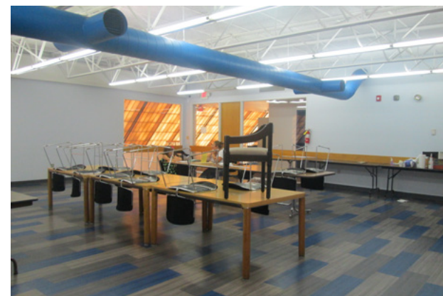
Upper Level Meeting Room
