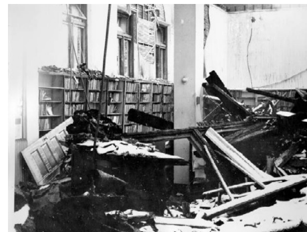
Extensive Fire Damage (original building) - 1957
